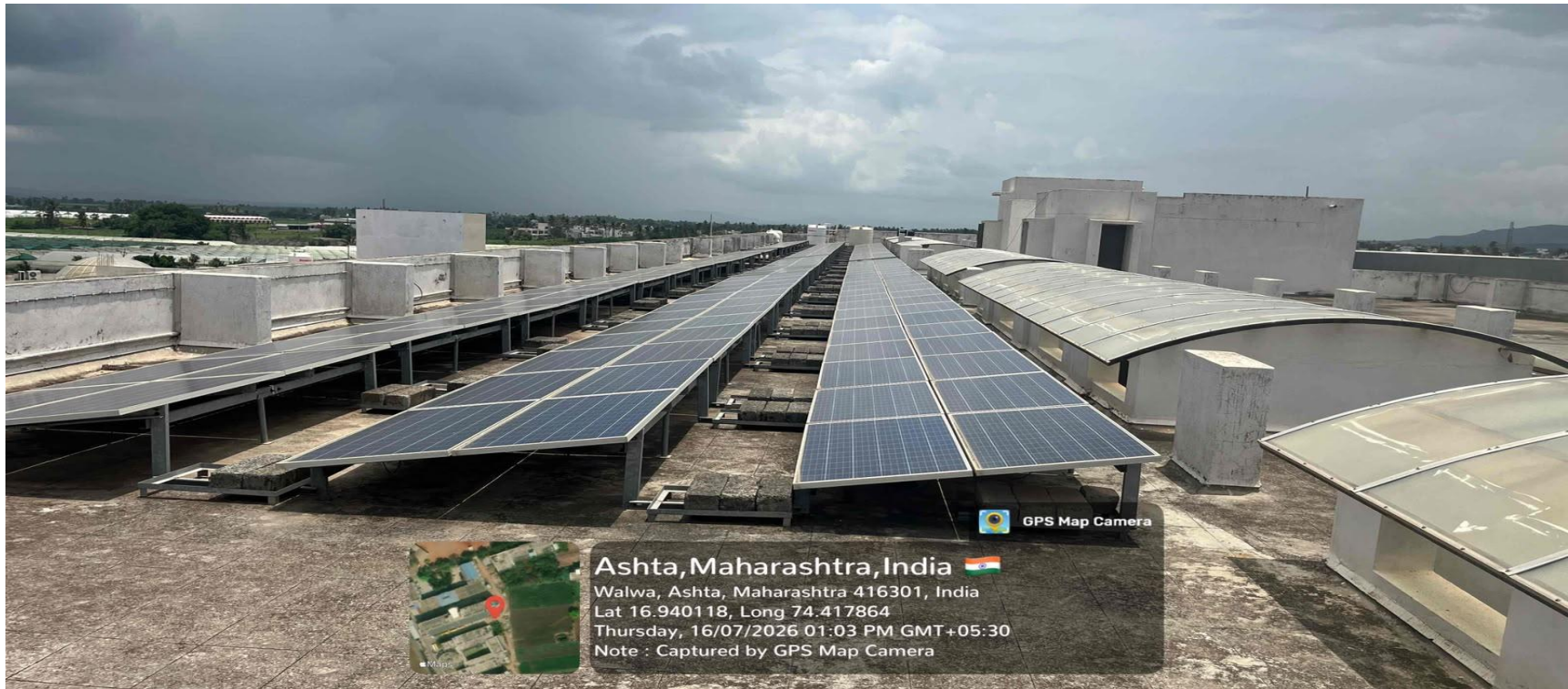
100 KW Solar power generation
