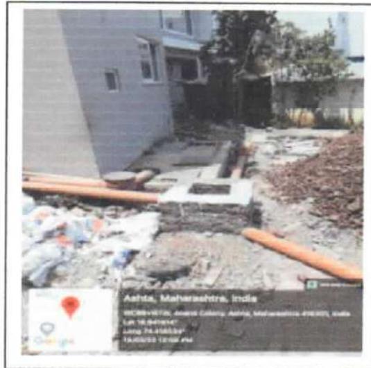
Rain water harvesting system
