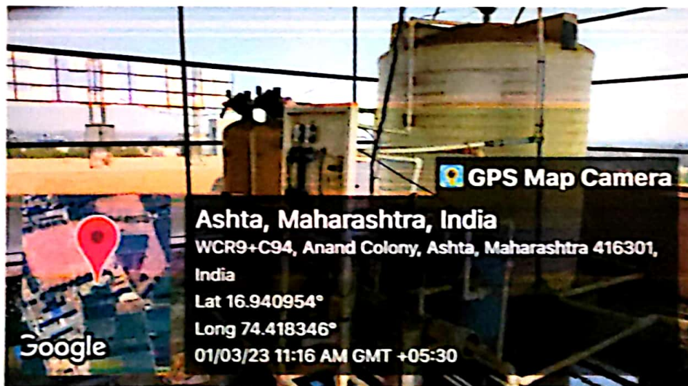
Fig 8.1: R.O. treatment plant for the campus (location: above Civil Engineering Department)
