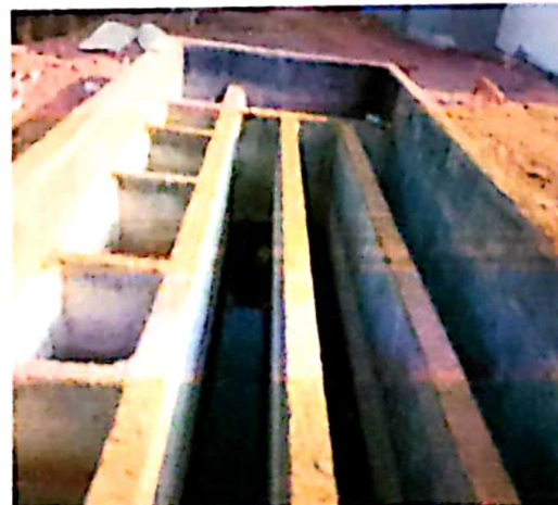
Fig 5: Waste water treatment facility in the campus
