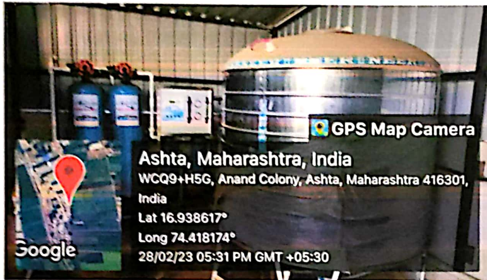
Fig 8.2: R.O. treatment plant for the hostel (location: above Ladies hostel)
