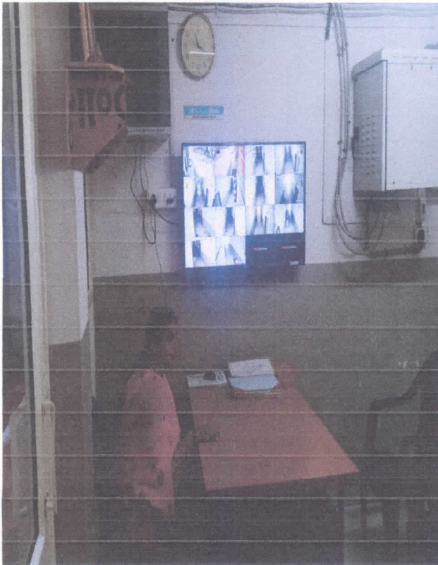
CCTV inLadies hosted building
